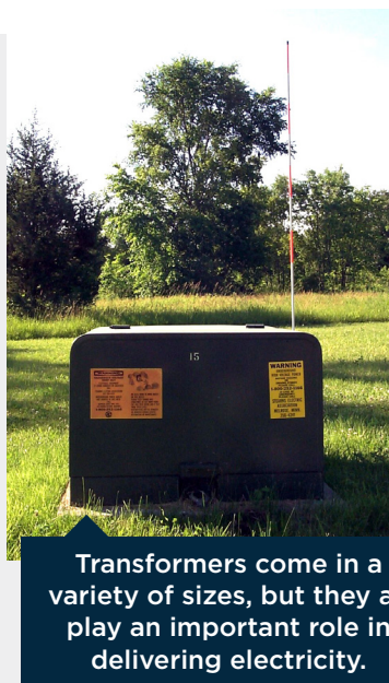
REA Linemen work to assure the new transformer at the Glenwood Substation sits properly on the concrete pad.
