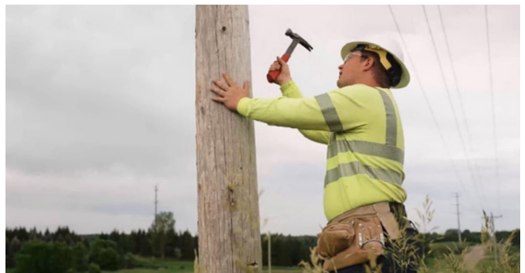
Sound inspections are done by hammering on all sides of the pole. The hammering produces a sound that can indicate if decay is present in the pole.
