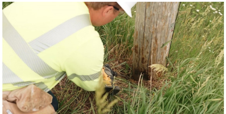
Boring inspections are done by drilling a hole into the pole at a 45-degree angle below the groundline. Wood shavings and any voids that the drill hits will indicate if any decay is present.
