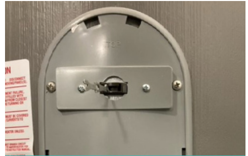
The lower element disconnect in the ON position. (To the left)
