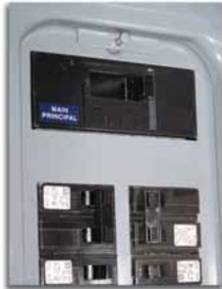
In this service panel, the "main" is located on top. Learn where your main is located.
