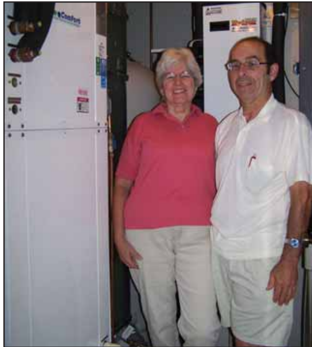
Today's heat pumps are compact compared to earlier models. Dian and Andy Lopez's utility room holds their geothermal heatpumps, plus a Marathon water heater.
